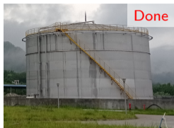
5000 m 3 LAB tank
