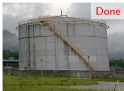
5000 m 3 LAB tank
