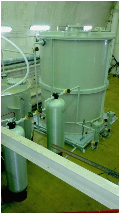
Water purification system
